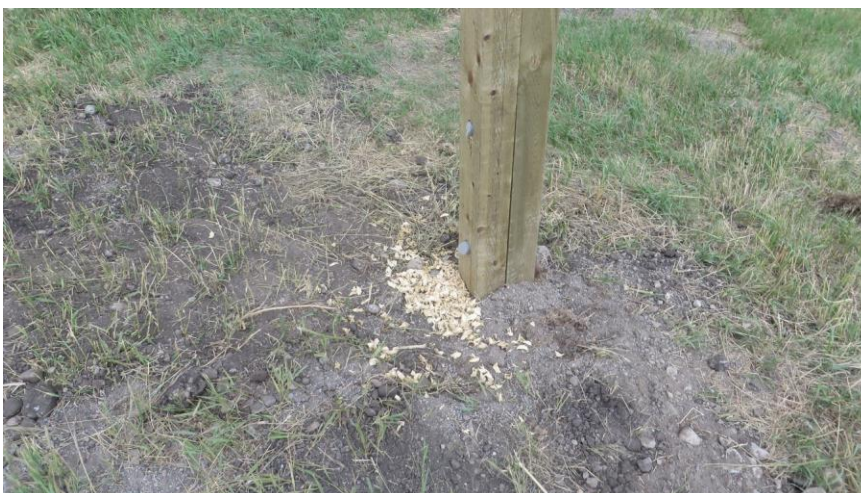
The double-wide post for the Stop sign and flashing red light on the east approach.
