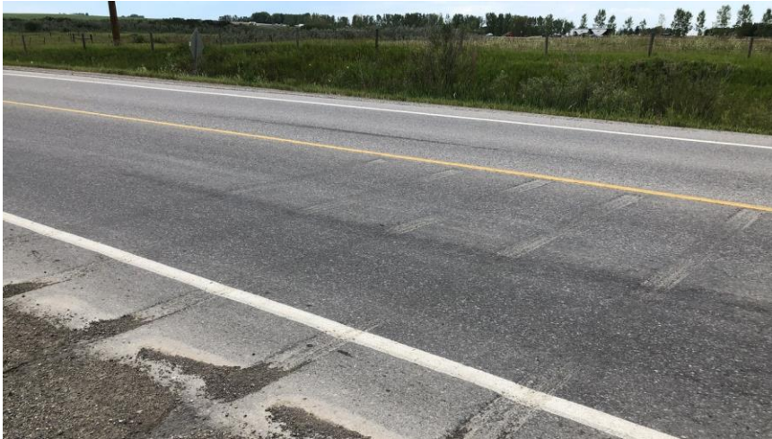
Transverse rumble strips on the west approach are worn in the wheel paths.
