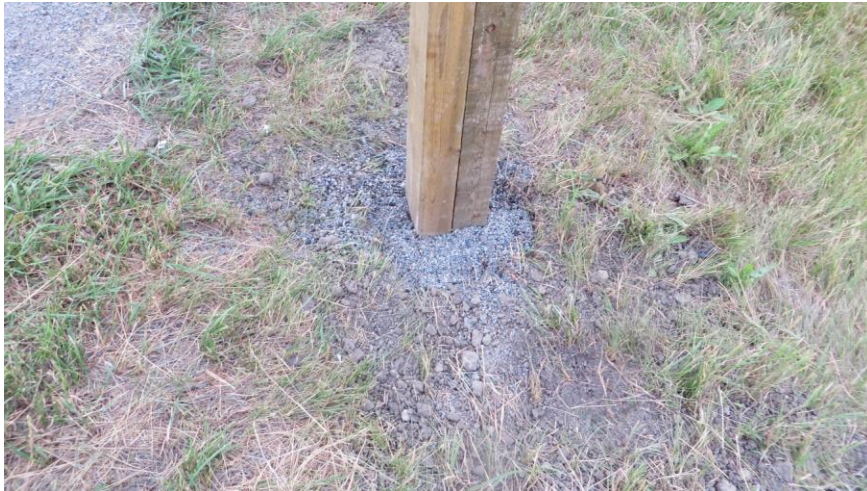
The double-wide post for the Stop sign and flashing red light on the west approach.
