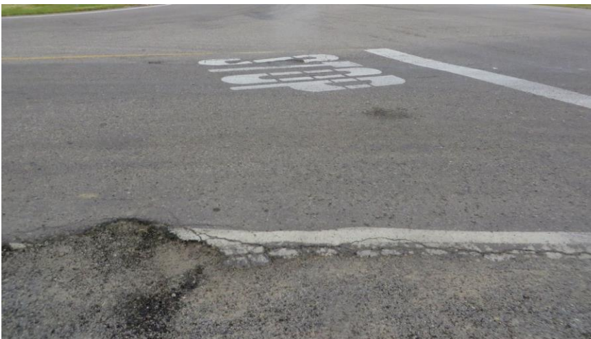
Pavement deterioration on the south edge of the west approach.
