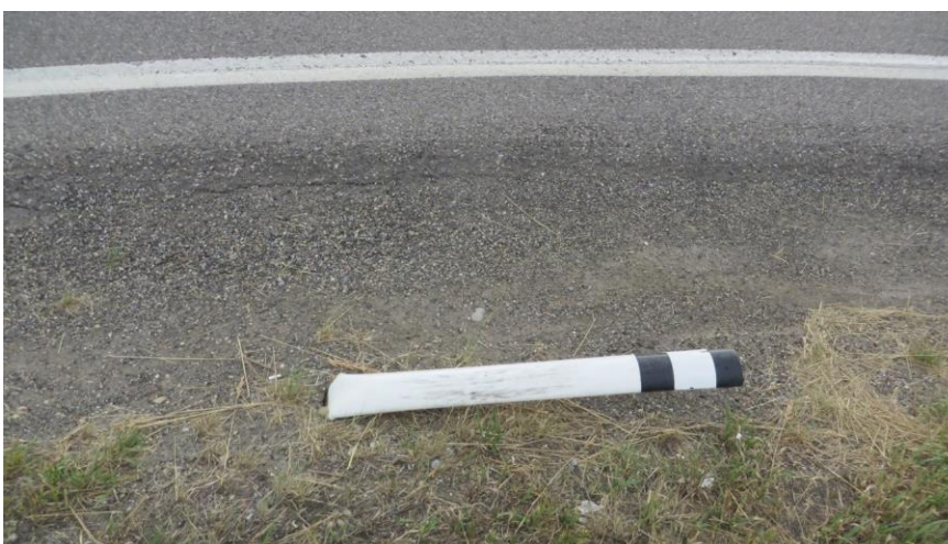
A delineator guide post beside the southbound right turn radius was bent over / flattened.
