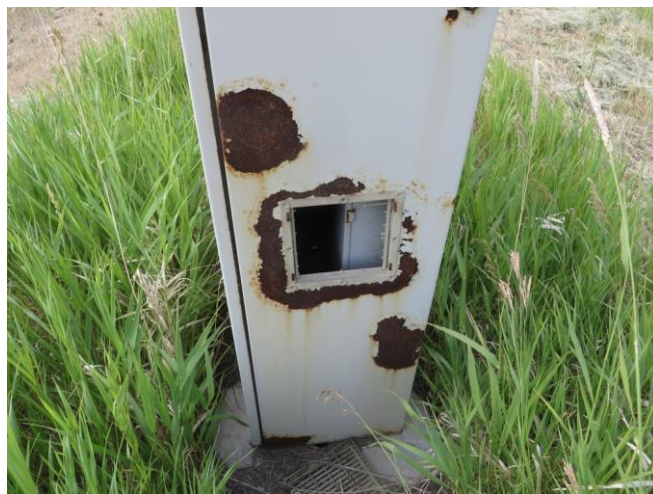
Missing access louvre on the side of the illumination system PDC.
