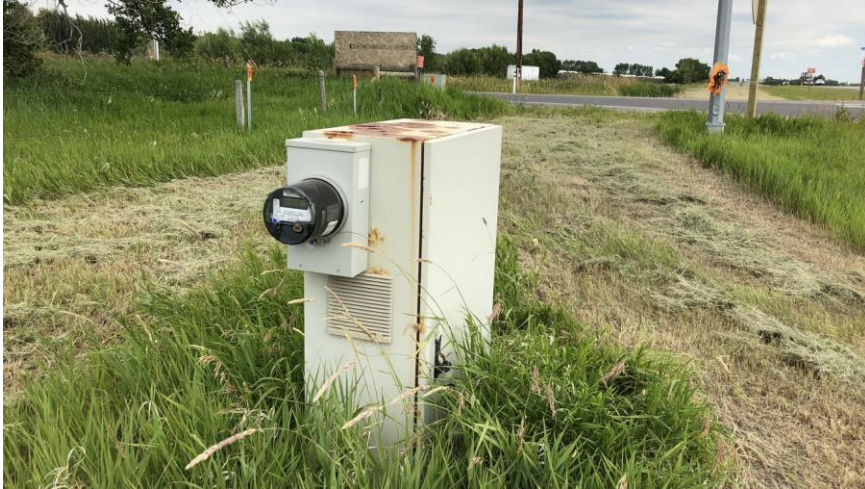
The power distribution cabinet (PDC) for the illumination system.
