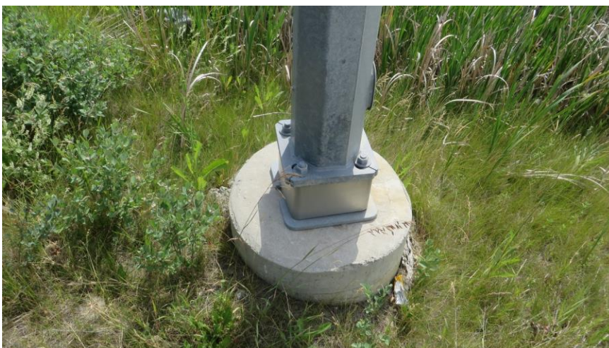
Street light pole base in southeast corner of intersection (Pole#17035338).
