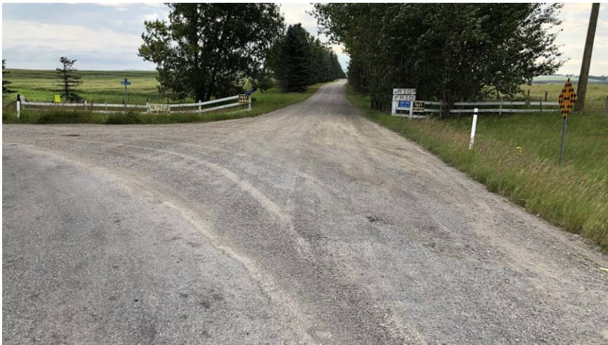
The east leg of the TR204/RR291 intersection functions as a multi-parcel country residential access.
