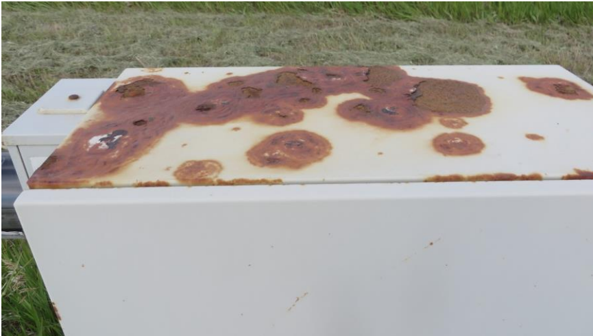
Rust on top of the illumination system PDC.
