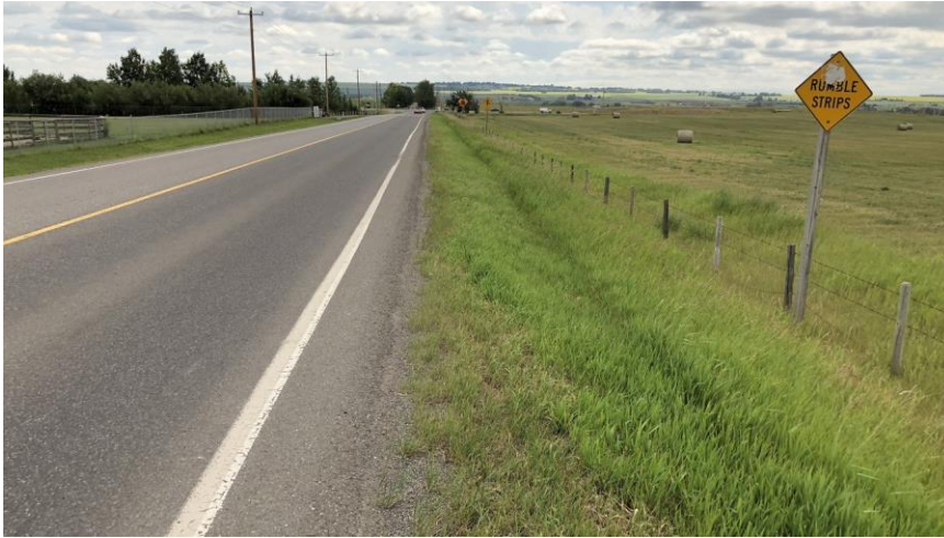
Looking toward the intersection from the Rumble Strips sign on the west approach.
