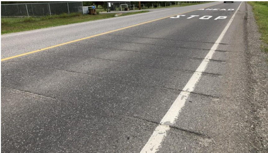
Transverse rumble strips on the west approach are worn in the wheel paths.
